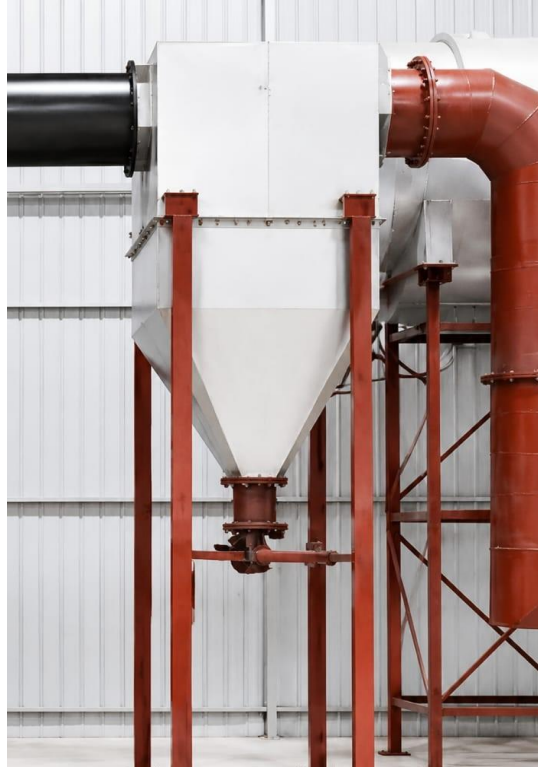
Mechanical dust collector
